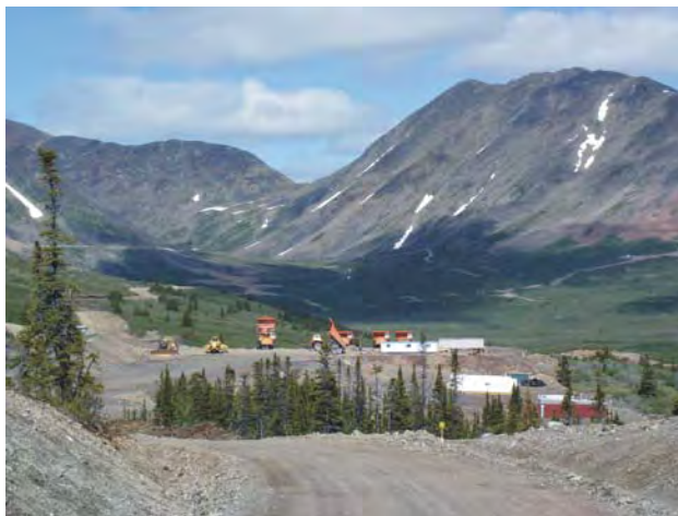
Figure 1.10. Ruby Creek, construction equipment parked on the new mine access road; tailings site in the distance.
