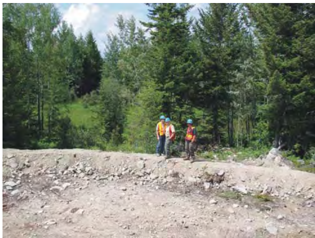
Figure 3.12. Drill pad reclamation at Gibraltar. (The barrier is to prevent runoff into the nearby wetland.)
