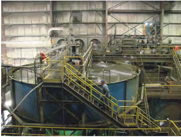
Figure 3.4. Filtration tank, Mount Polley Mine Mill.
